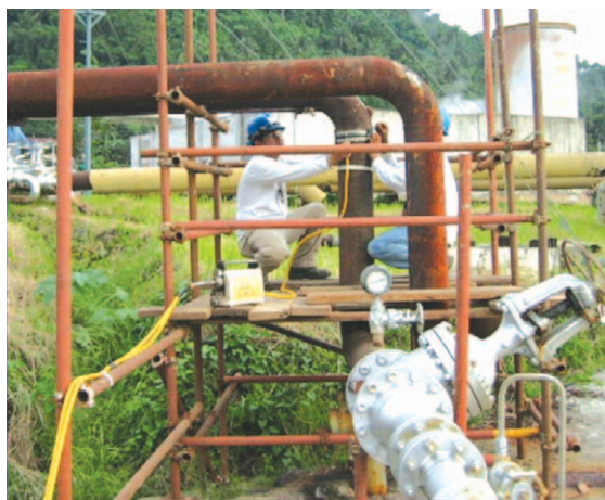
Radiographic Testing of Newly Constructed Pipeline in the Philippine Geothermal Power Plant
